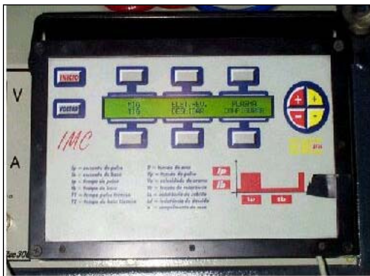
Figura 20. Panel de control
