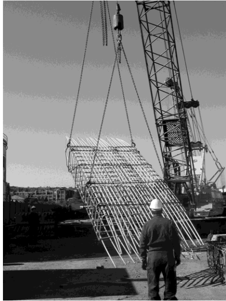
Figure 1.3. Reinforcing cage being readied for placement in forms for a tunneling application.
