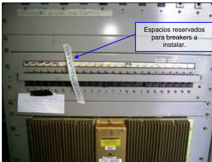
Panel de Breakers @-48Vdc
