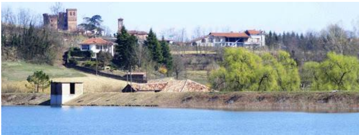
Figure 2. Picture of the embankment and the concrete structure enclosing the pipeline. Extracted from PiemonteParchi, (n.d.).
