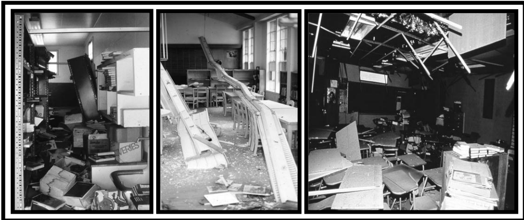
Figura 8. Desprendimiento o volcamiento de elementos no estructurales. Tomadas de Design Guide for Improving School Safety in Earthquakes, Floods, and High Winds. Risk Management Series. FEMA 424 (de izq. a der., Figs.4-10,4-12,4-27, pp.4-17,4-19,4-30 respect.) de Arnold, Lyons, Munger, Quinn y Smith, 2004, enero, Washington, DC.
